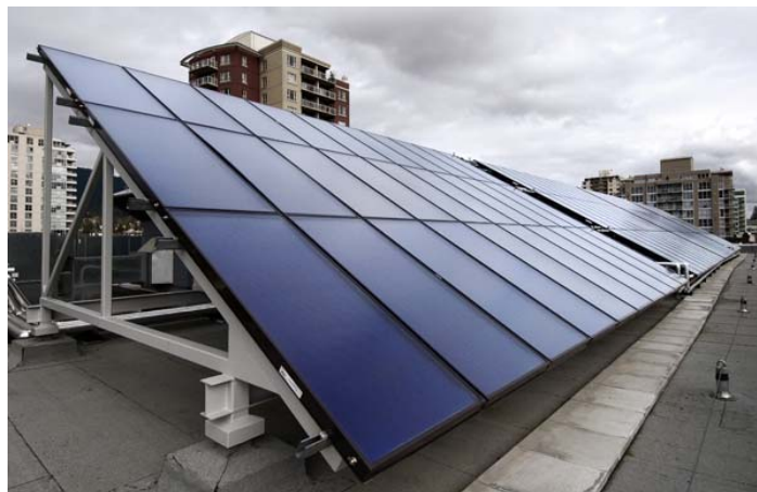
Figure 14 - Solar Hot Water Panels - North Vancouver
