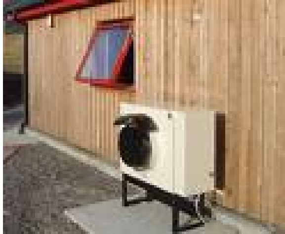
Figure 14 - Air Source Heat Pump
